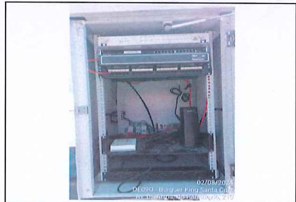
Foto 117 Interior do Rack Shelter
