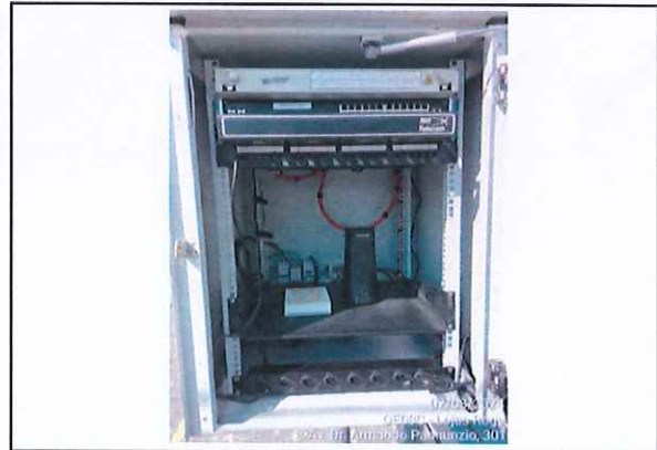
Foto 37 Interior do Rack Shelter
