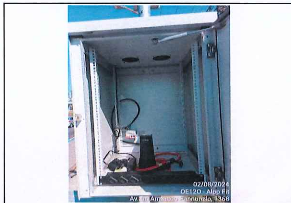
Foto 134 Interior do Rack Shelter
