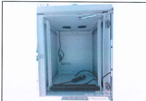
Foto 43 Interior do Rack Shelter
