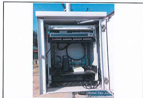
Foto 55 Interior do Rack Shelter
