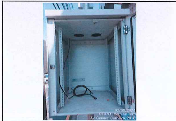
Foto 106 Interior do Rack Shelter
