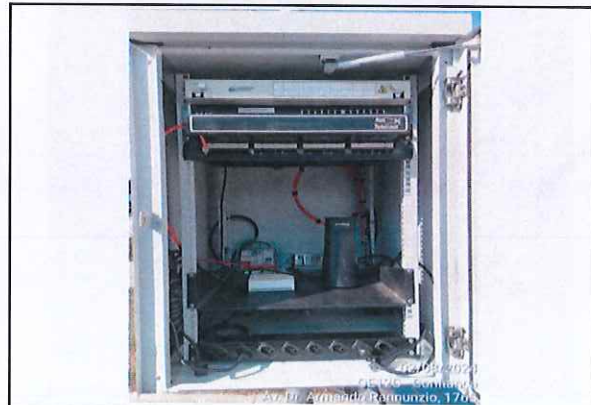
Foto 63 Interior do Rack Shelter
