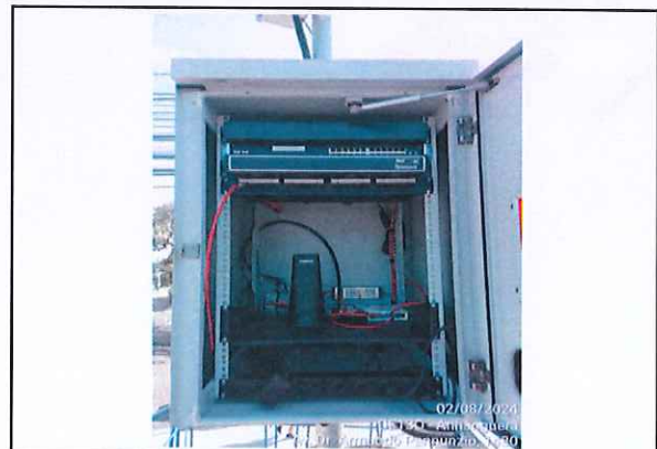
Foto 140 Interior do Rack Shelter
