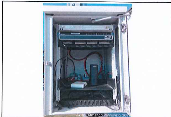
Foto 69 Interior do Rack Shelter
