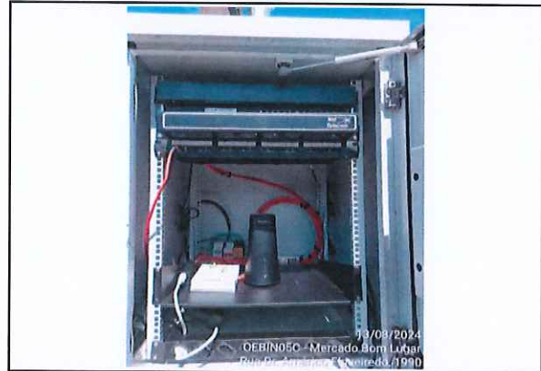
Foto 179 Interior do Rack Shelter
