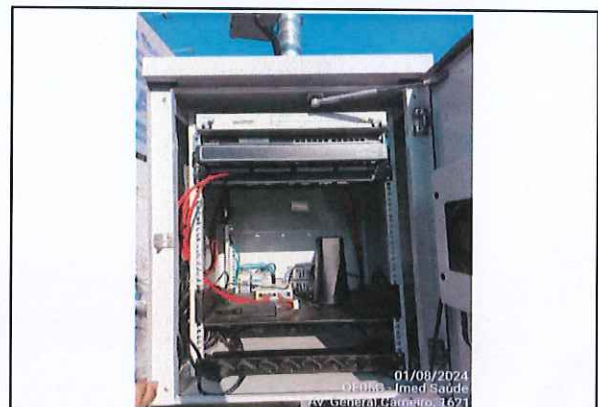
Foto 19 Interior do Rack Shelter
