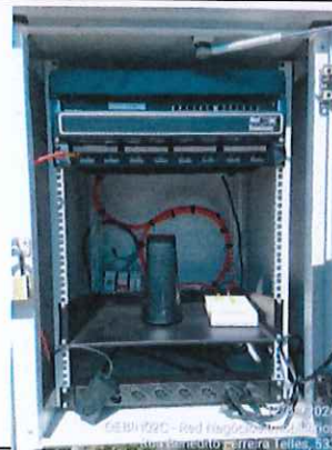
Foto 197 Interior do Rack Shelter
