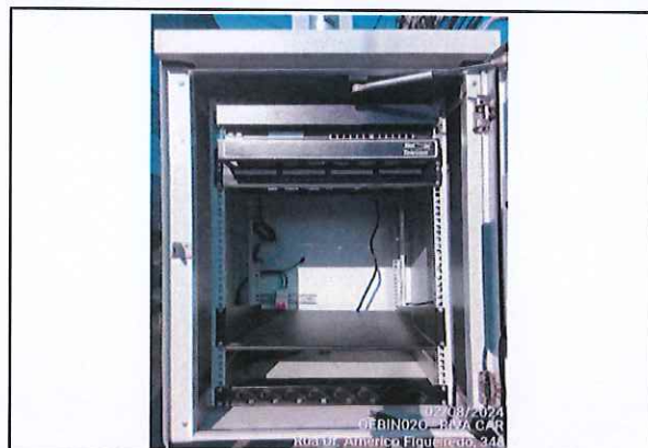
Foto 157 Interior do Rack Shelter
