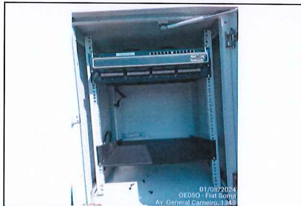
Foto 93 Interior do Rack Shelter
