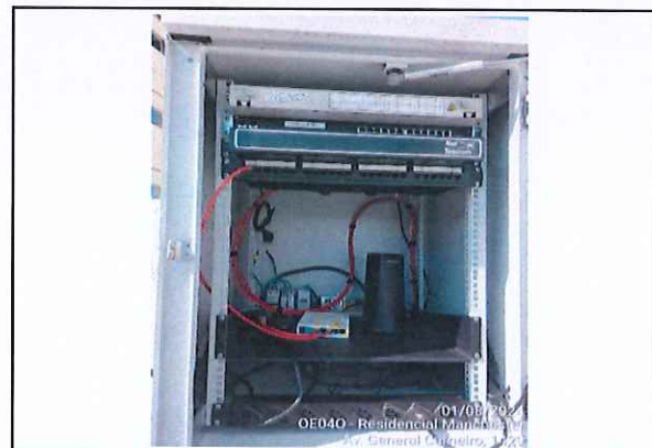
Foto 13 Interior do Rack Shelter
