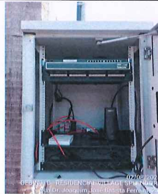
Foto 203 Interior do Rack Shelter
