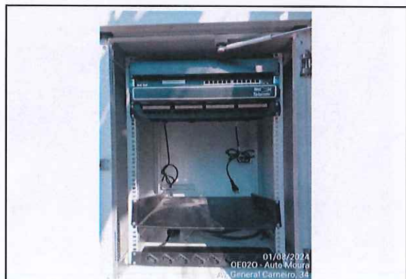
Foto 76 Interior do Rack Shelter
