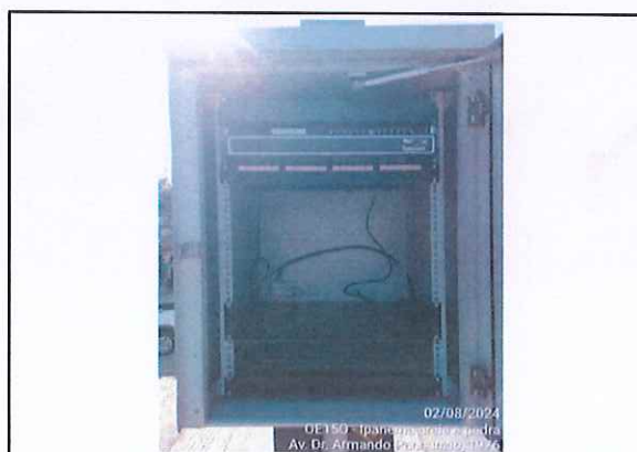
Foto 152 Interior do Rack Shelter
