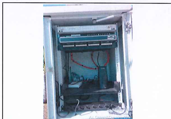
Foto 25 Interior do Rack Shelter
