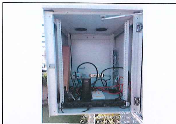
Foto 146 Interior do Rack Shelter
