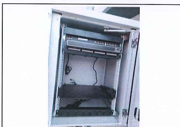
Foto 81 Interior do Rack Shelter
