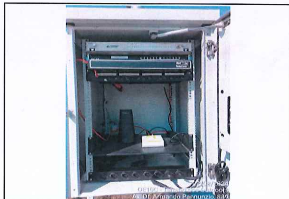
Foto 49 Interior do Rack Shelter
