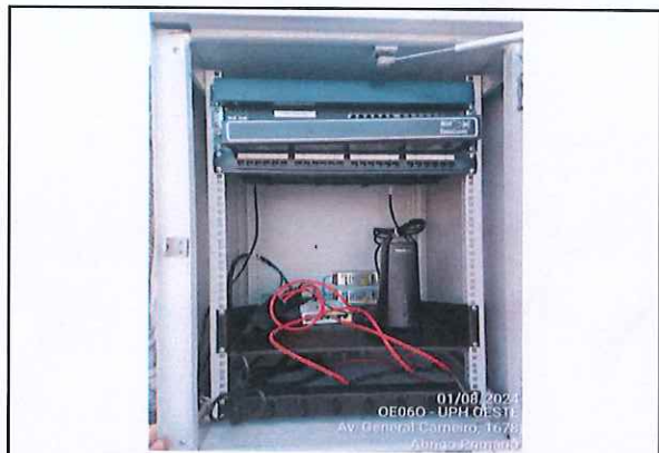
Foto 98 Interior do Rack Shelter
